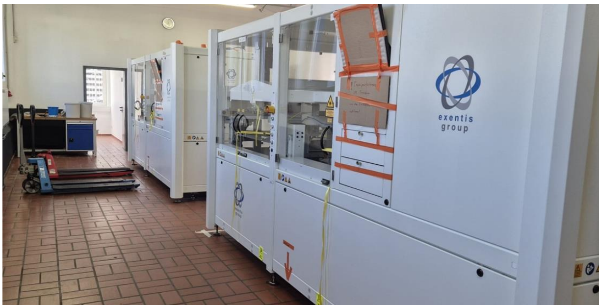
Installation of two Exentis 3D production systems at Whitecell's production site in Clausthal-Zellerfeld
